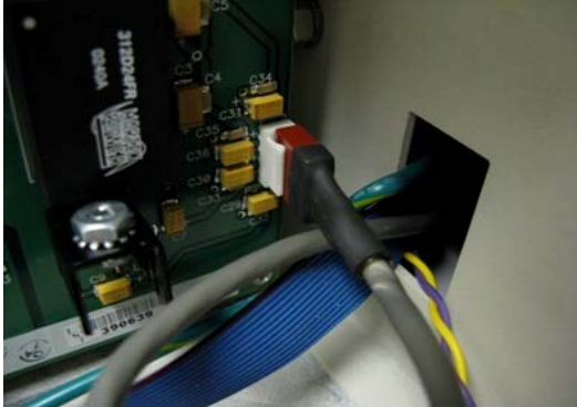
The gray, five conductor cable.
