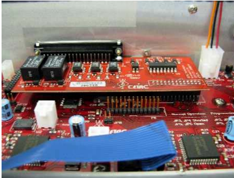
Figure 1-17. Main and Daughter board replaced in system.
